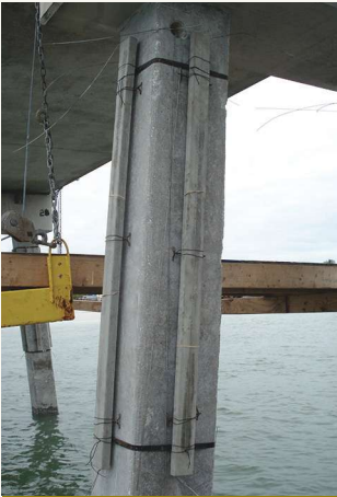
Figure 6. Dry jacket that includes alkali-activated anodes on the pile prior to jacketing (bulk zinc anode not shown).
