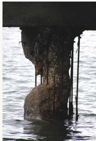
Figure 1. Corrosion of prestressed pile in tidal/splash zone. All Photos and Figures: Vector Corrosion.
