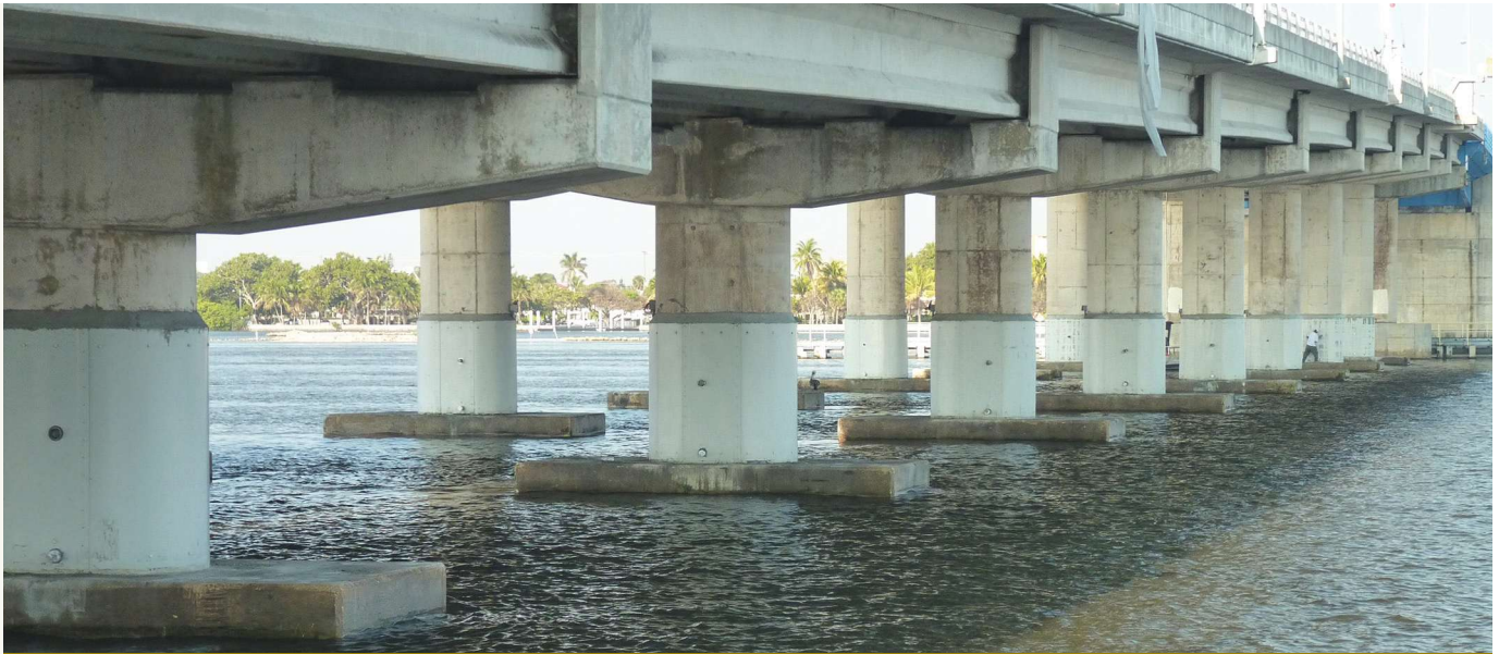
Figure 5. Installed dry jacket system that includes galvanic jackets with activated anodes (no bulk anodes).
